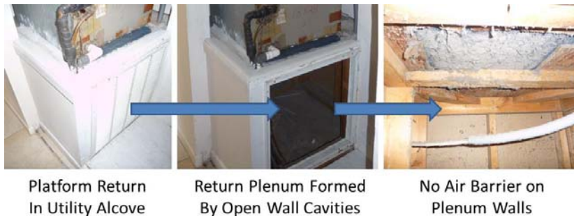
Figure 1 – Return plenum formed by unfinished frame walls and air handler support platform in a utility alcove.
